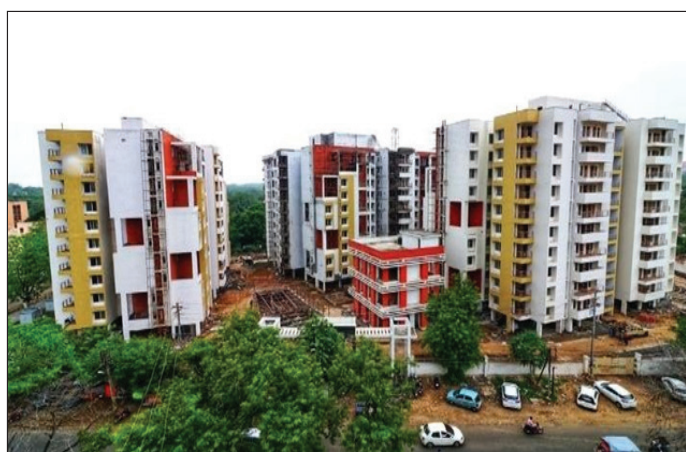
Construction of 222 Flats at Keelandev Tower, Bhopal for MP Housing & Infrastructure Development Board.
