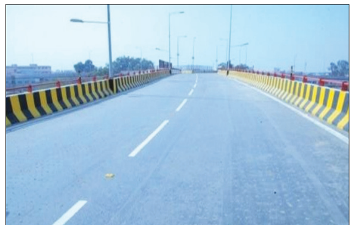
Construction of 2 lane Railway overbridge at Sonapat for Haryana State Roads and Bridges Development Corporation Ltd.
