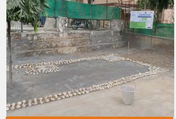
Rain Water Harvesting Structure – B 4 Vasant Kunj
