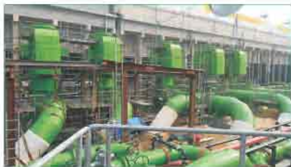
Successful Commissioning of Marubeni a/c South Bangkok Power Plant Project, Thailand
