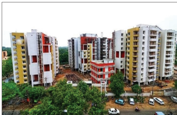
Construction of 222 Flats at Keelandev Tower, Bhopal for MP Housing & Infrastructure Development Board.
