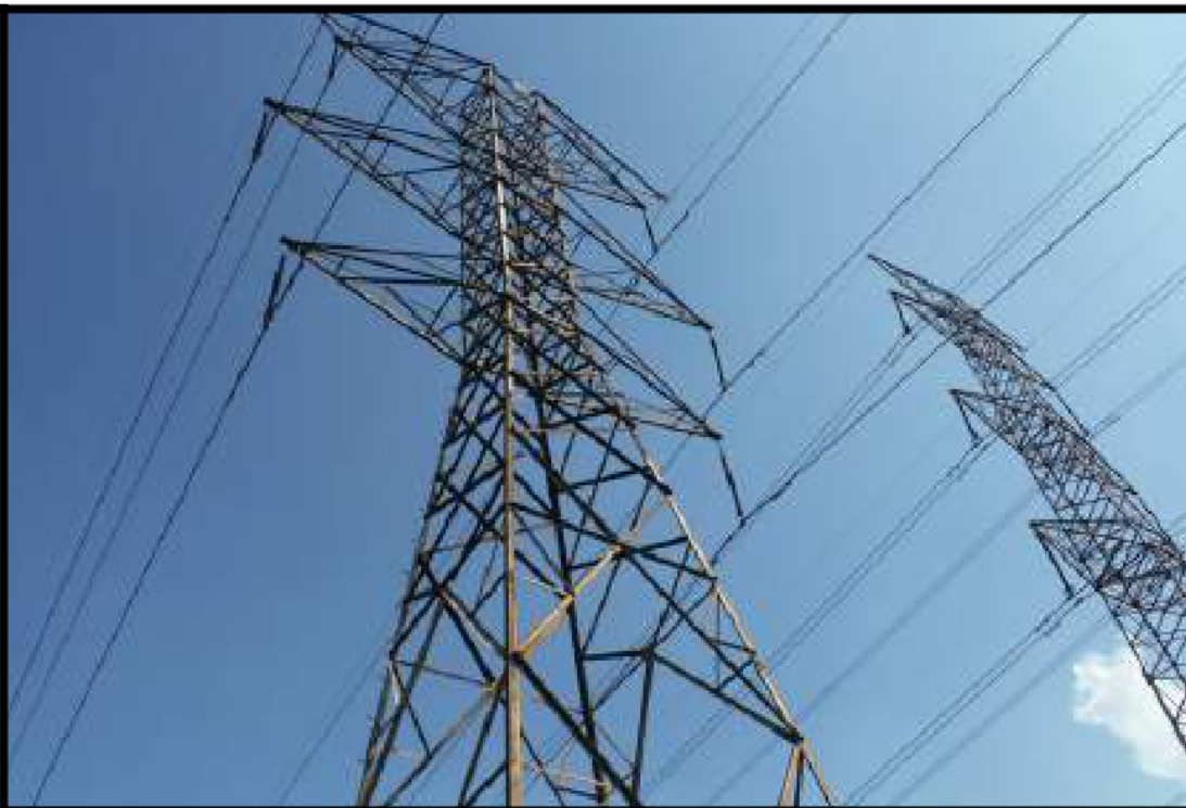
Pictures from Advait Plant, Kadi (Mehsana) in Gujarat
