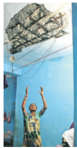
A resident points to the slab fell off at her house in a colony in Jeevan Nagar in Vadodara. Bhupendra Rana
