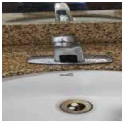
Use of Water tap sensors
