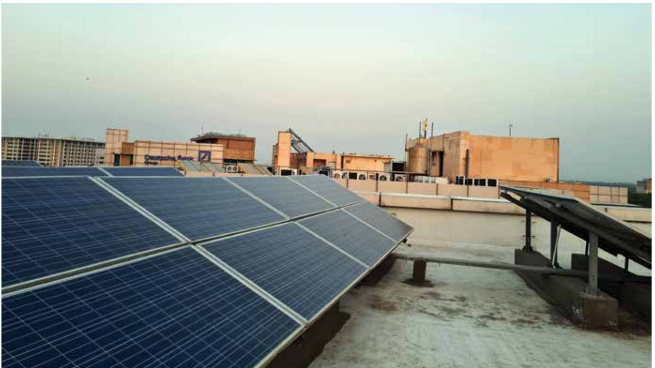
210 kWp - Rooftop Solar, @Evolve, Mahindra World City, Jaipur
