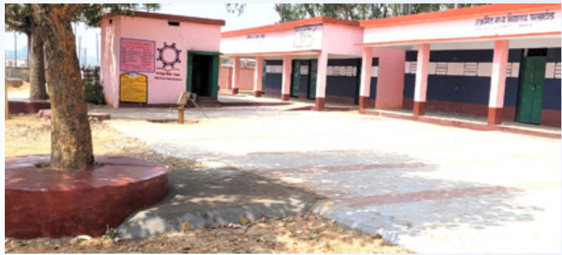
Finishing of Repair and Renovation works at Utkramita Madhya Vidyalaya, Giridih, Jharkhand under CSR
