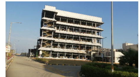
Specialty Fluorochemicals facility (Dahej, India)
