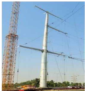
765kV S/C Monopole
