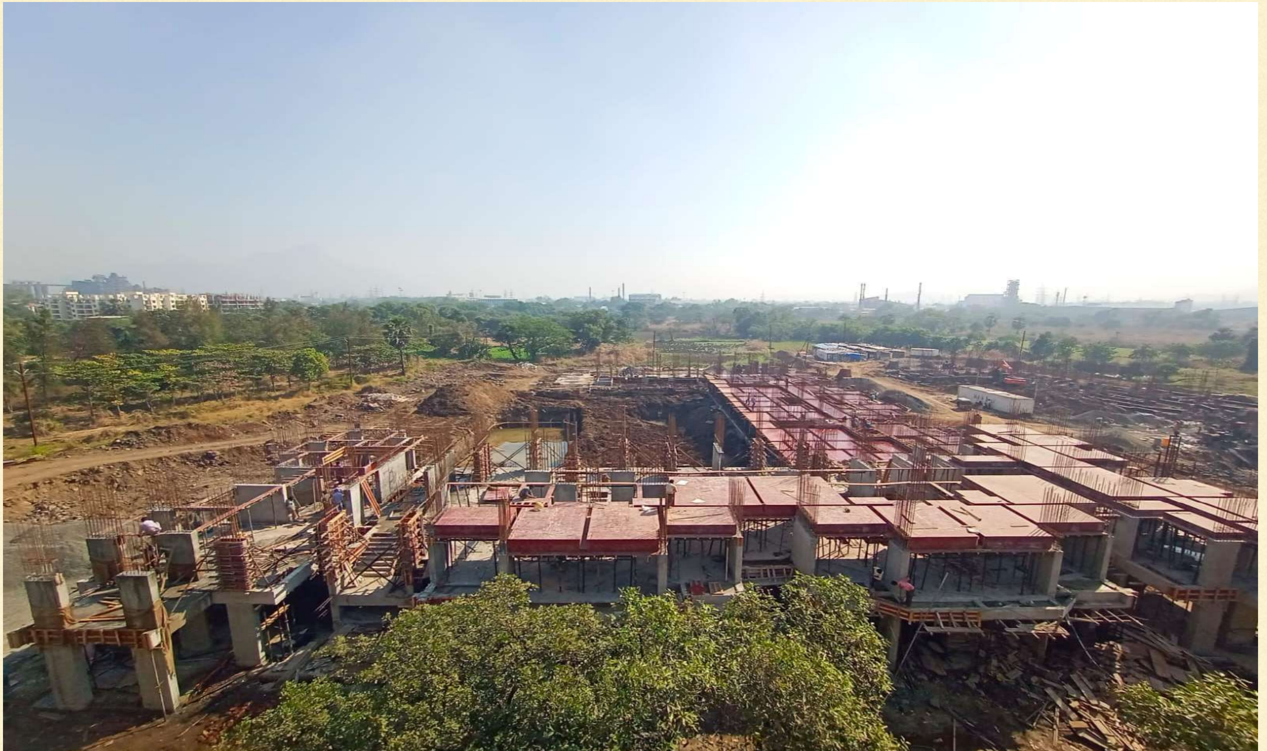
Slab work in progress for R & S wing, Plinth work in progress for T wing
