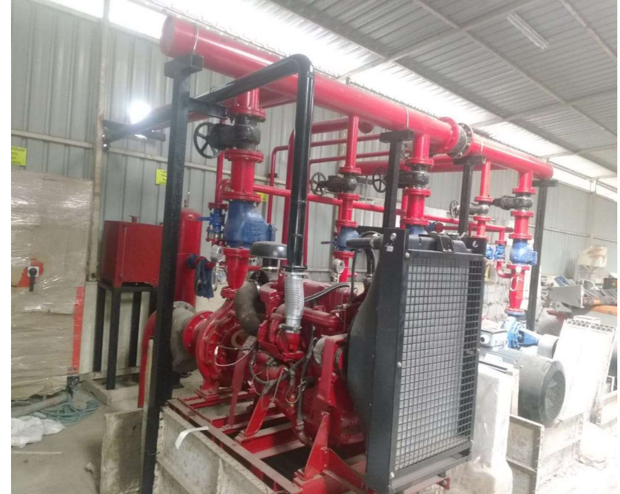
Fire Fighting Systems installed at Siyaram Textiles, Amravati
