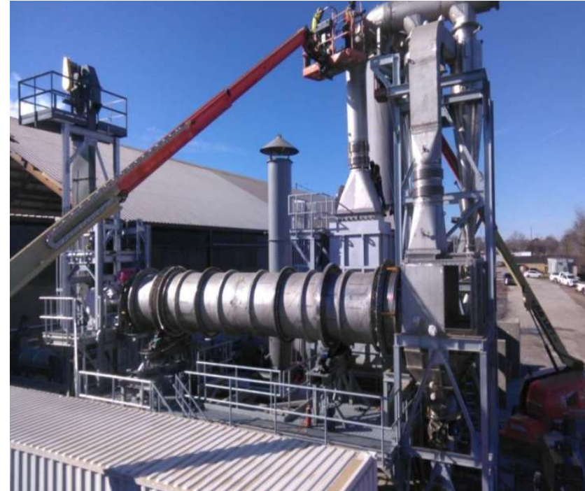
Torreactor drum assembly for Torrefaction plant, TSI USA
