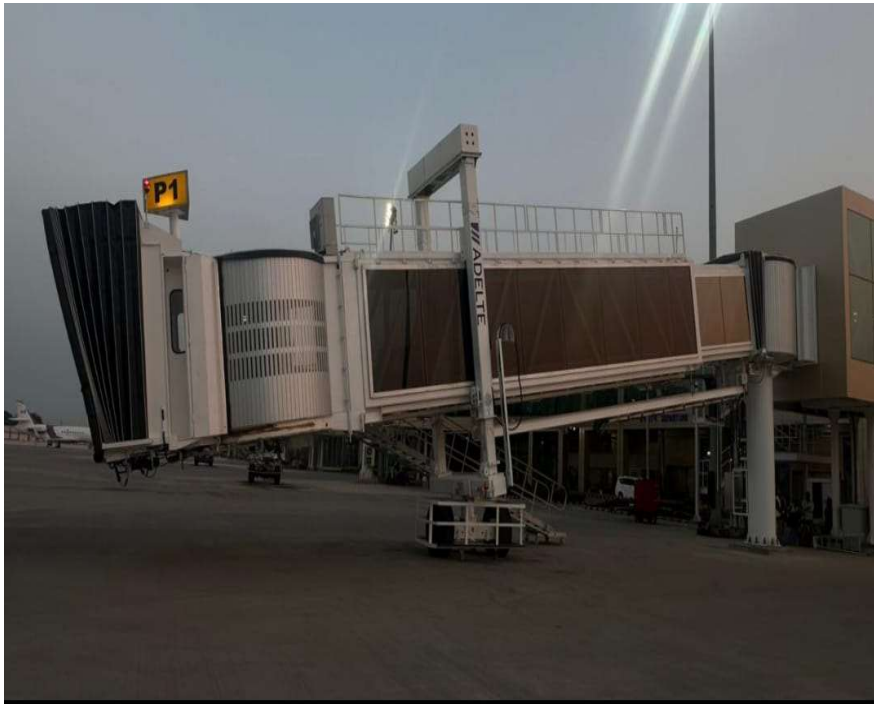
Passenger Boarding Bridge Installed at Prayagraj Airport
