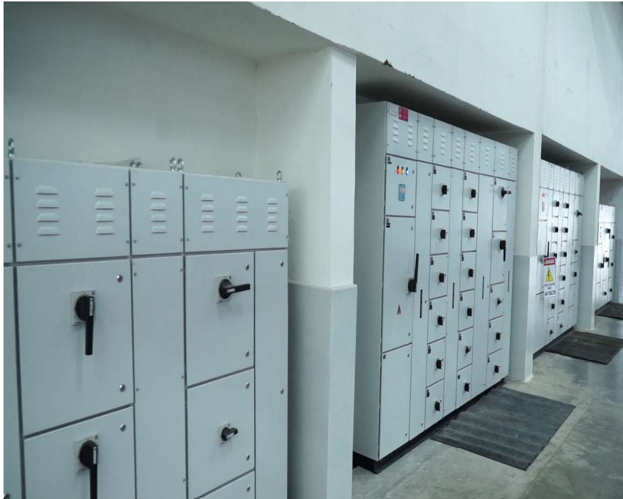
Electrical Panel Supplied for Spinning Mill Bhagirathi Textile, Nagpur
