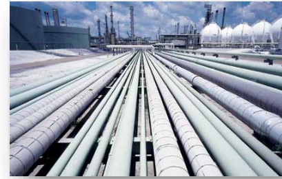
Anti Corrosive Material
