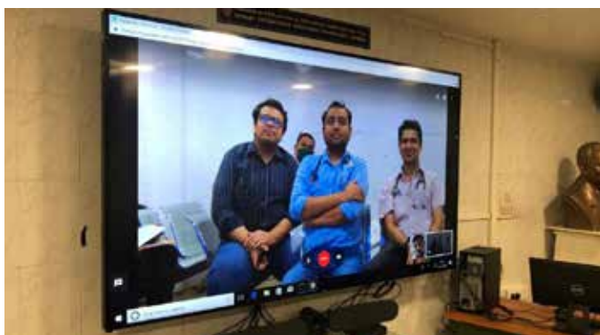
State-of-the-art video conferencing system installed at K E M. Hospital, Parel, Mumbai
