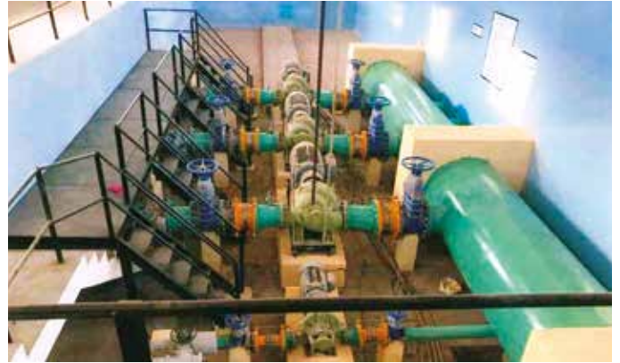
Installation of Pumping Machineries at Scheme No. 8 under Alwar NCR, in Rajasthan.
