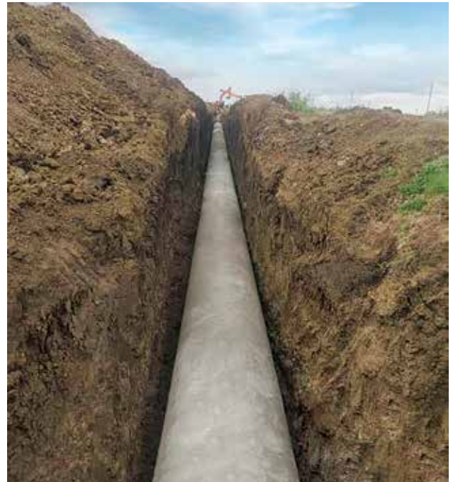
1250 mm dia MS pipeline laying at Kushtagi MI & GWDD project, in Karnataka.
