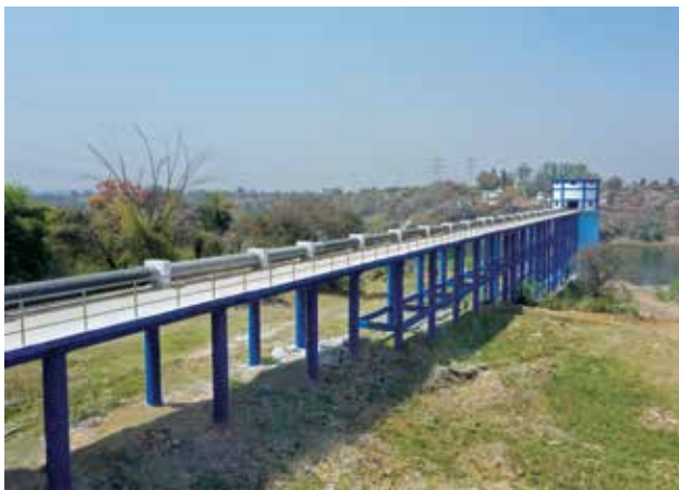
Intake well cum pump house at Bhedaghat Town, for Bhedaghat Water Supply Scheme, in Madhya Pradesh.
