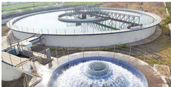
Clarifloculator & Aerator for 31 MLD water treatment plant for Jalgaon Jamod Water Supply Scheme, in Maharashtra
