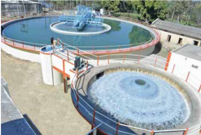
25.5 MLD Water Treatment Plant at Ashoknagar Road for Guna Water Supply Project, in Madhya Pradesh.
