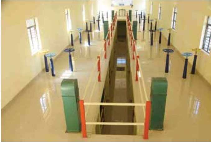
25.5 MLD Water Treatment Plant Filter House for Guna Water Supply Project, in Madhya Pradesh.
