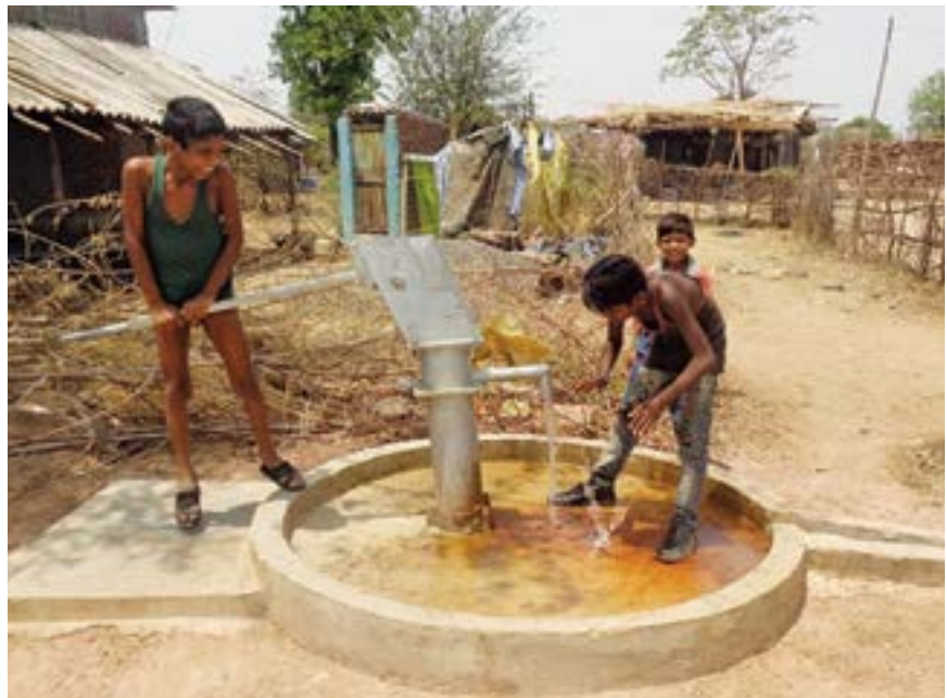
One of the handpump installed in a village, Budhni (MP)
