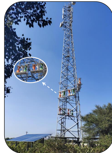
Solar & Wind powered Site solution
