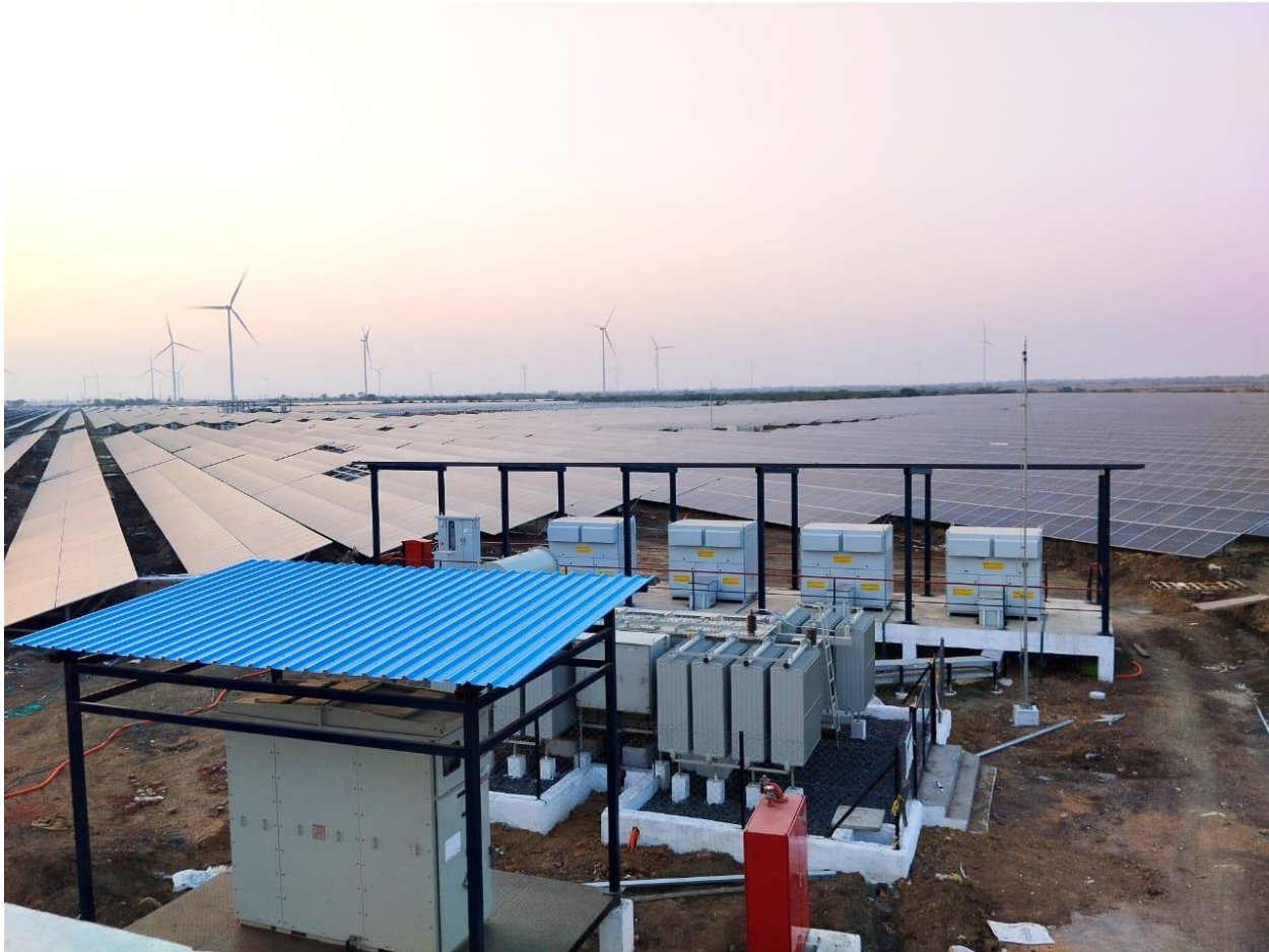
Figure 1 The 160 MW solar ground-mounted site at Bhavnagar, Gujarat
