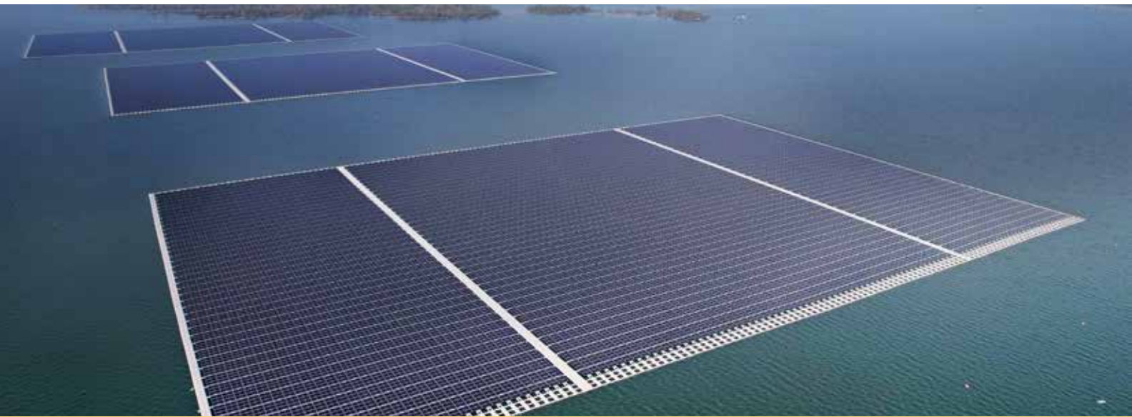
90 MW Floating Solar Project, Omkareshwar, Madhya Pradesh
