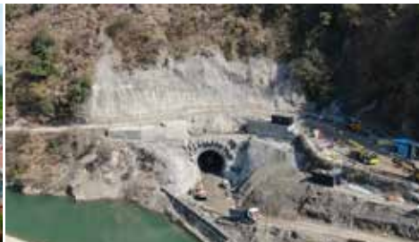
Hydro Power Plant
