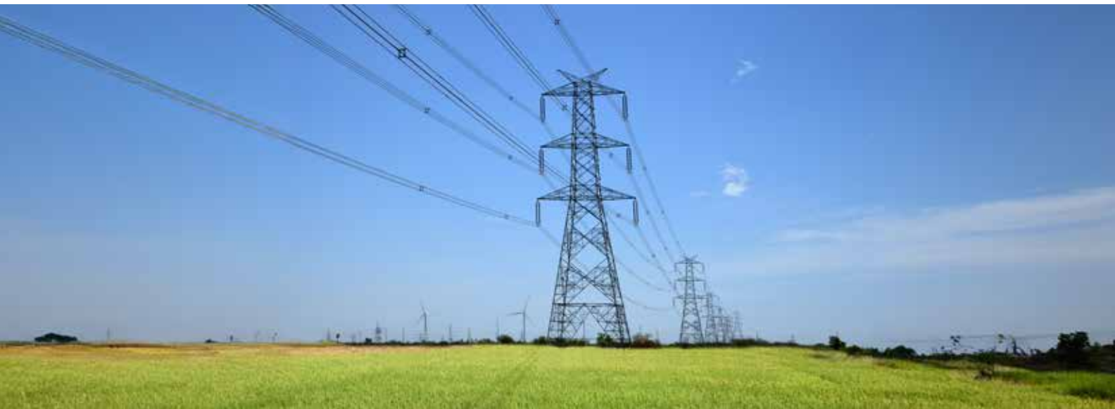
400kV Ottapidaram, Tamil Nadu
