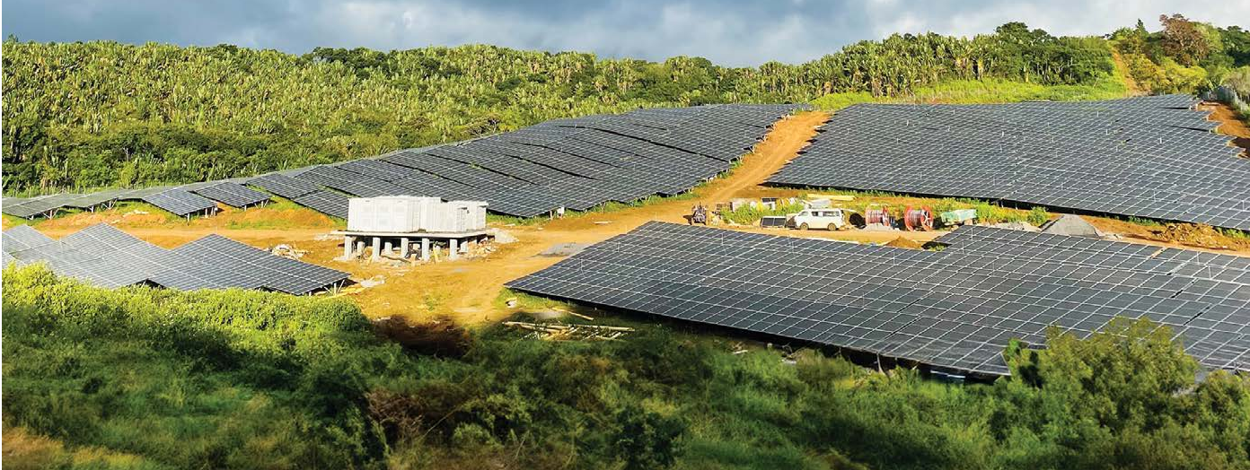
8 MW ac Tamarind Fall Solar PV Project in Henrietta, Mauritius commissioned by BHEL
