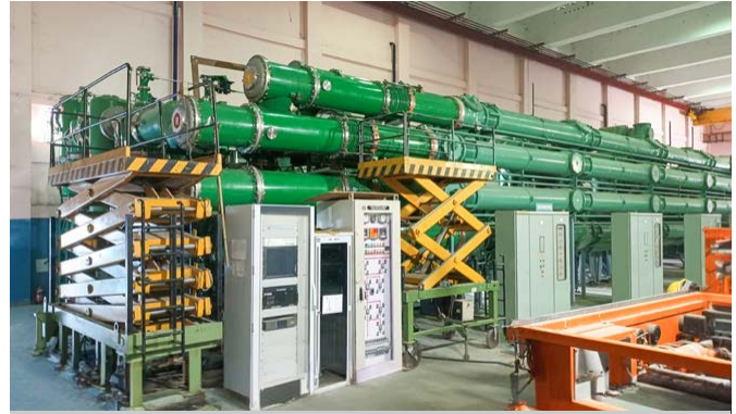
400kV Gas Insulated Switchgear (GIS) bay at Chamera HEP indigenously developed by BHEL under the Aatmanirbhar Bharat initiative
