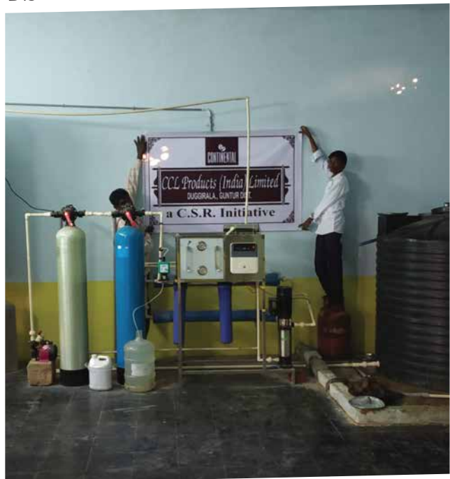
Providing RO drinking water units
