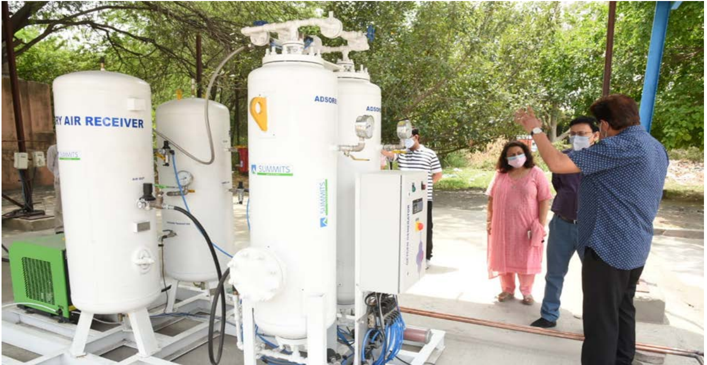
Oxygen Generation Plant installed by NTPC
