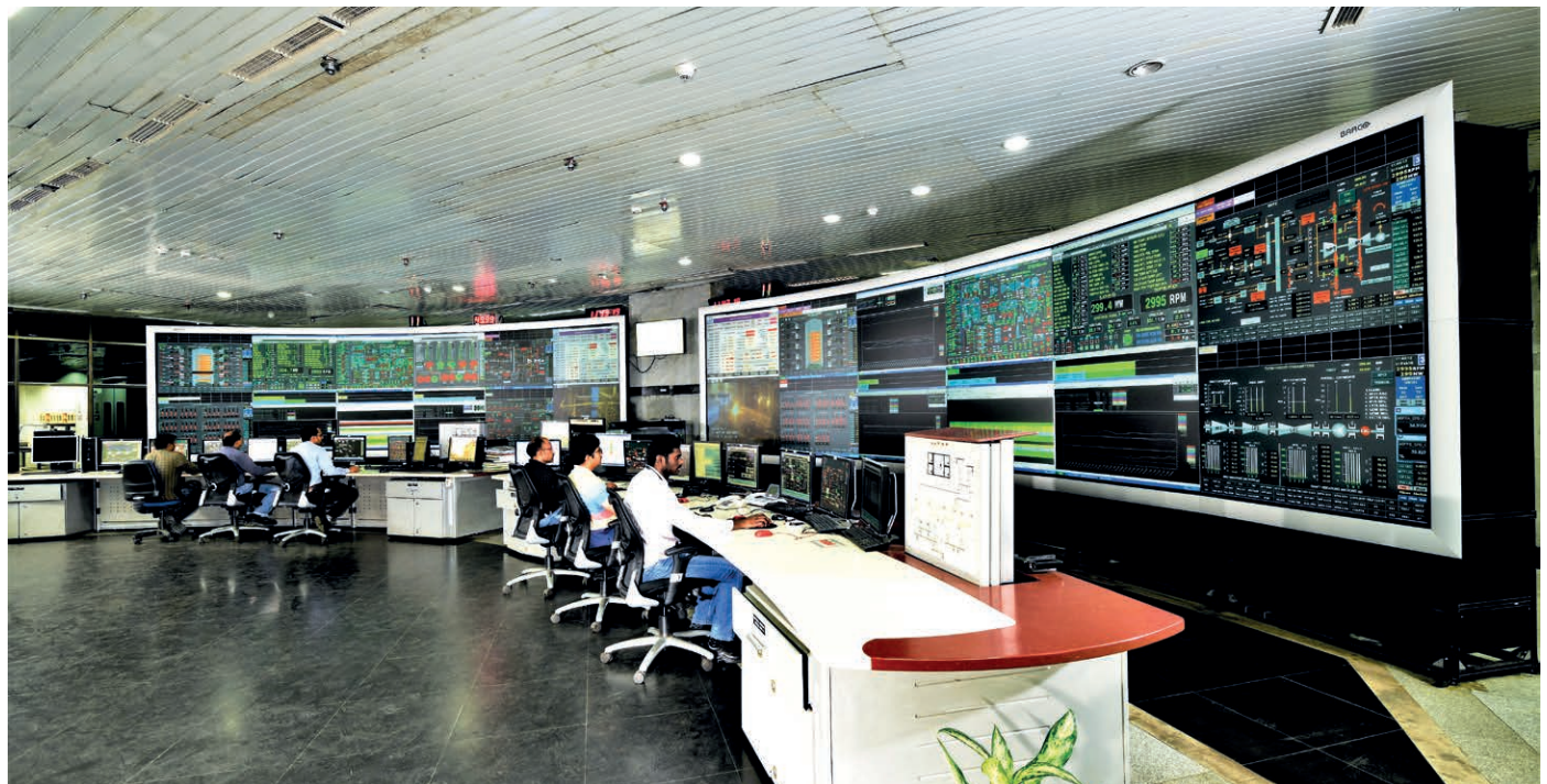
Control Room at NTPC Bongaigaon
