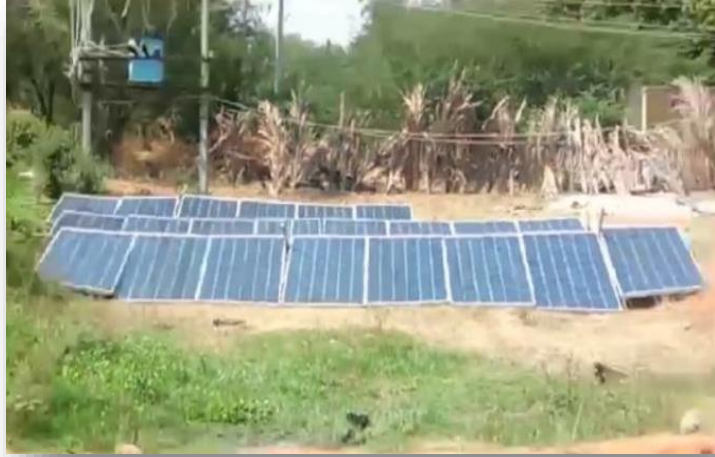
Shakti Solar SCR Pumps Model : 9000 Watt Discharge : 327,000 LPD (India)
