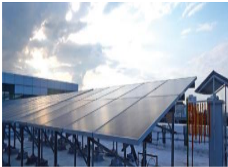
Roof-top solar plant
