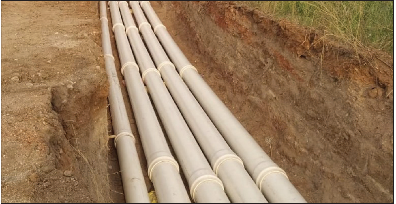
PVCO Pipes laying at Morepalayam Lift Irrigation Project and Sree Sivashakthi Lift Irrigation Project
