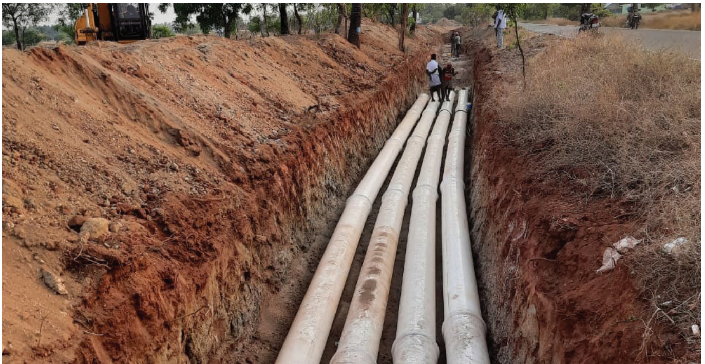
PVCO Pipes laying at Sri Arthanareeswarer Lift Irrigation Project and Sri Ponkalamman Lift Irrigation Project
