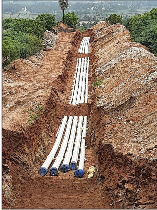
PVCO Pipes Laying at Morepalayam Lift Irrigation Project and Sree Sivashakthi Lift Irrigation Project
