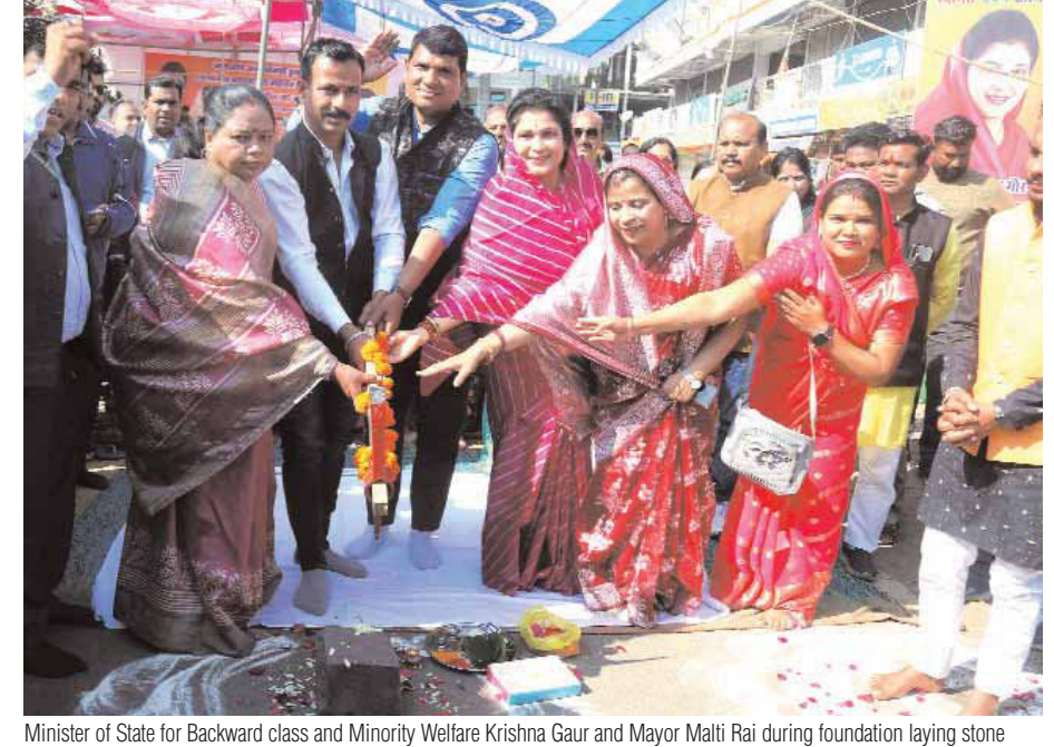
Minister of State for Backward class and Minority Welfare Krishna Gaur and Mayor Malti Rai during foundation laying stone ceremony for the drainage construction work in Govindpura locality in Bhopal on Friday. Pioneer photo
