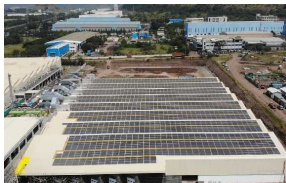
Solar Panels on Roof
