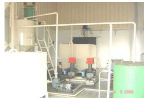
Effluent Treatment Plant
