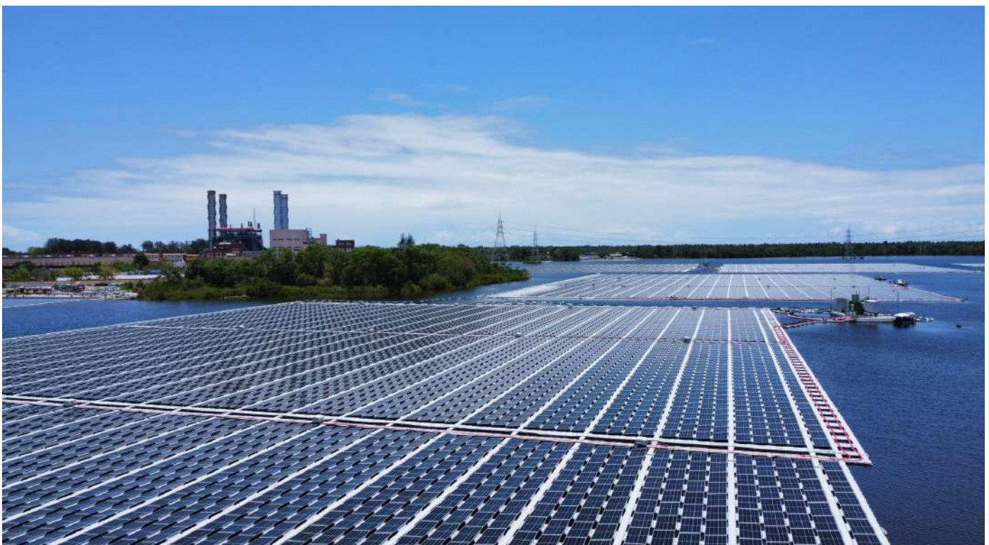
Floating Solar NTPC Kayamkulam
