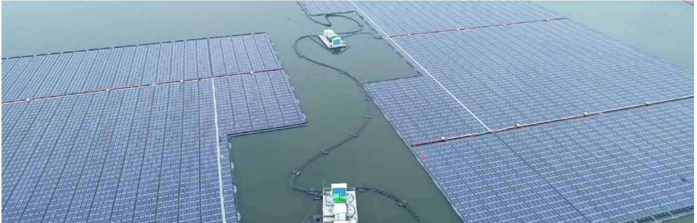
NTPC Ramagundam Floating Solar
