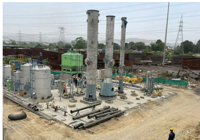
20 TPD Carbon Capture Plant, Vindhyachal
