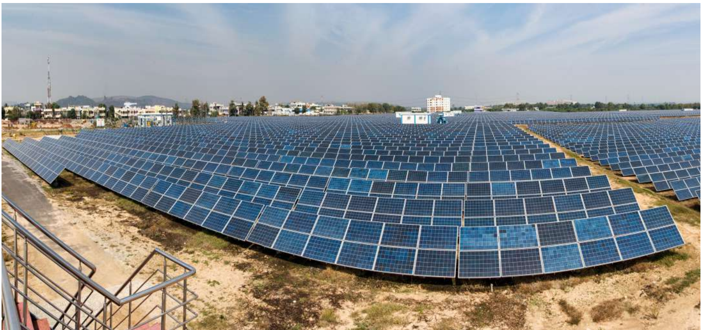
NTPC Solar at Ramagundam
