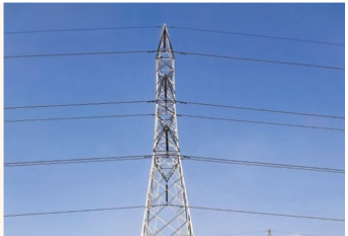
Transmission Tower at Surat
