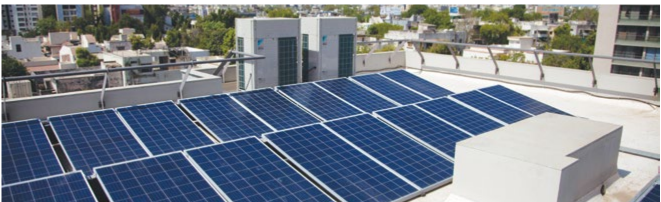
Captive Rooftop Solar System
