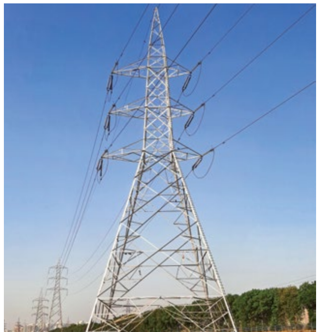
Transmission Tower at Surat
