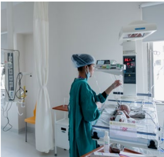
Well Equipped NICU and PICU facilities at UNM Children Hospital
