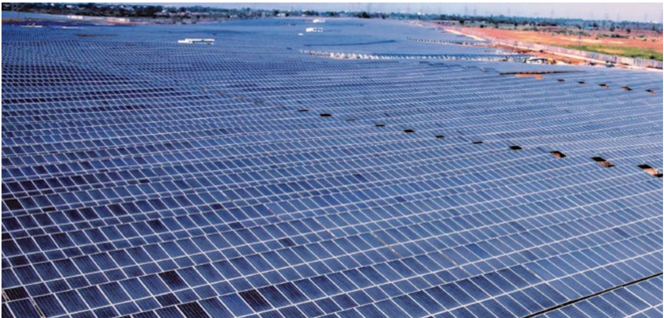
87 MW GENSU Solar Plant at Surat
