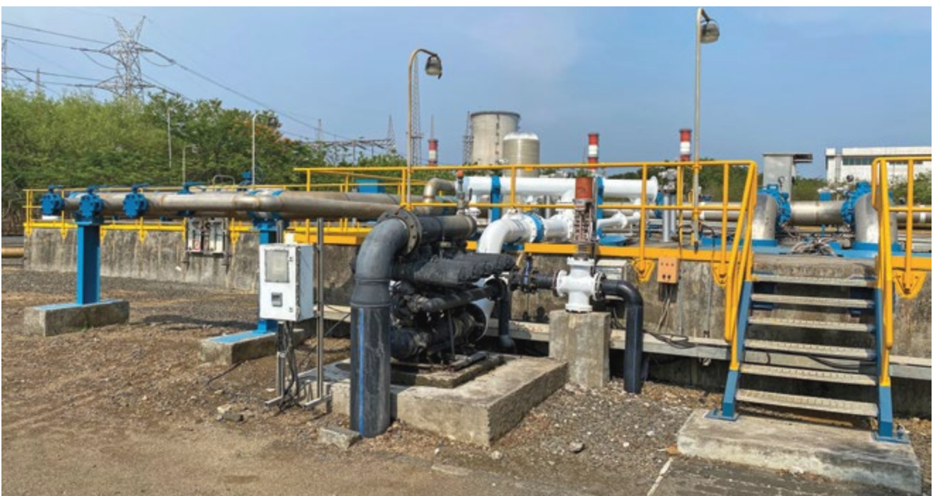
Efficient Water Management at SUGEN
