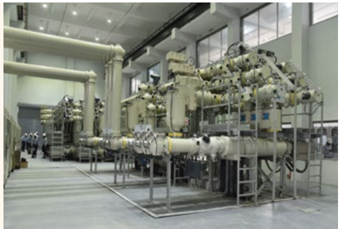
220 kV Substation at Gandhinagar
