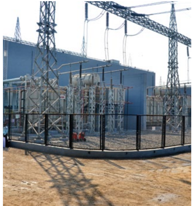
400 kV Nikol-2 Substation at Ahmedabad
