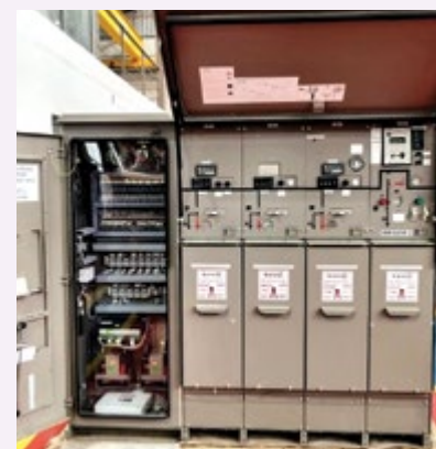
Distribution Automation Enabled Ring Main Unit (RMU)
