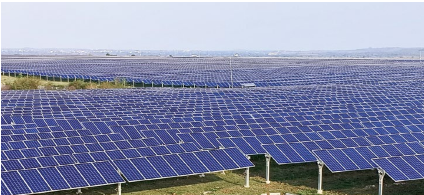
Our recently acquired 50 MW Solar Power Plant at Kamareddy, Telangana
