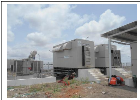
View of the solar power plant
