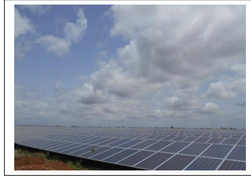
View of the solar power plant
