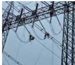
Sohna Substation Charging
