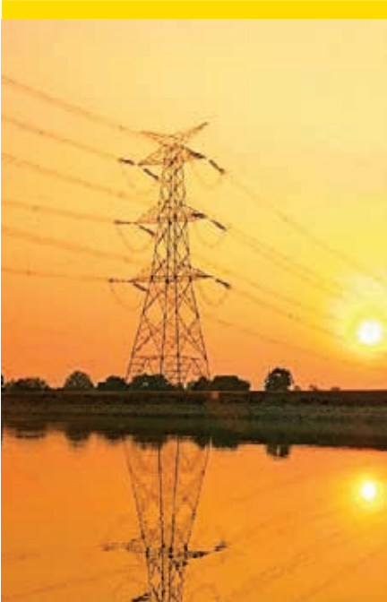
765 kV Vindhyachal-Jabalpur Transmission Line, Madhya Pradesh
