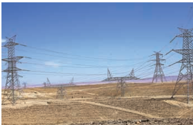
400 kV Al Qatrana-New Ma'an Transmission Line, Jordan
