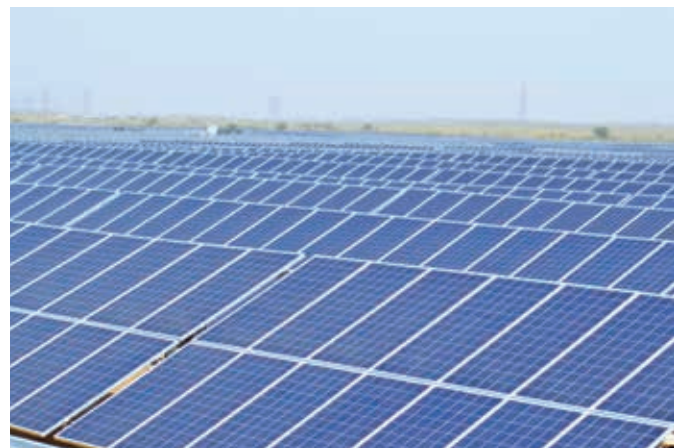
150 MWp Ground Mount Solar project for a leading domestic player
