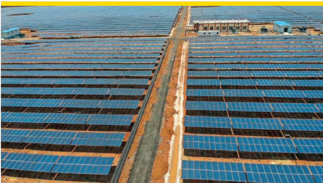
130 MWp Ground Mount Solar Project, Andhra Pradesh
