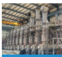
765/400 kV GIS Substation at Aligarh, Uttar Pradesh, dedicated to the nation by Hon'ble Prime Minister Shri Narendra Modi
