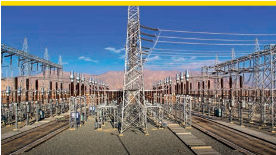
500/220 kV Dasht-e-Alwan AIS Substation at Pul-e-khumri, Afghanistan
