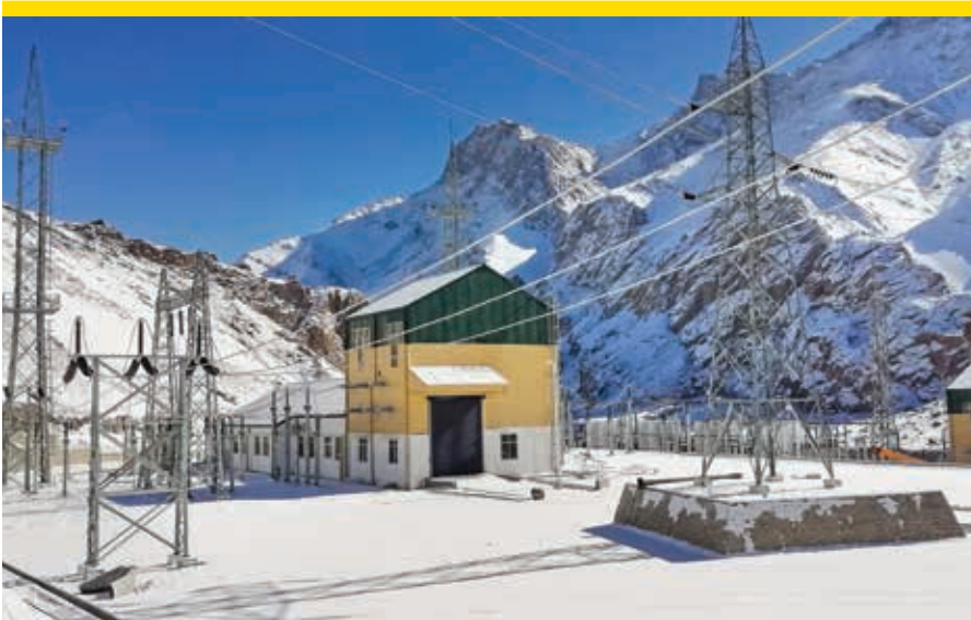
220/66 kV GIS Substation at Kargil & Drass, Jammu & Kashmir
