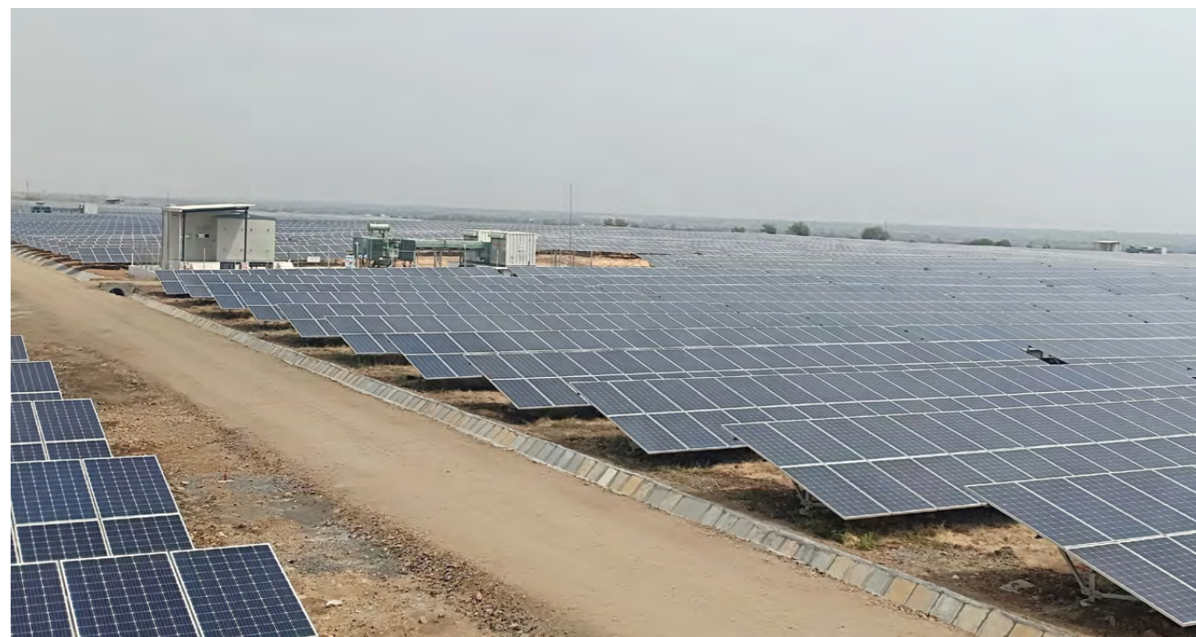
Our recently acquired 50 MW Solar Power Project at Solapur, Maharashtra
