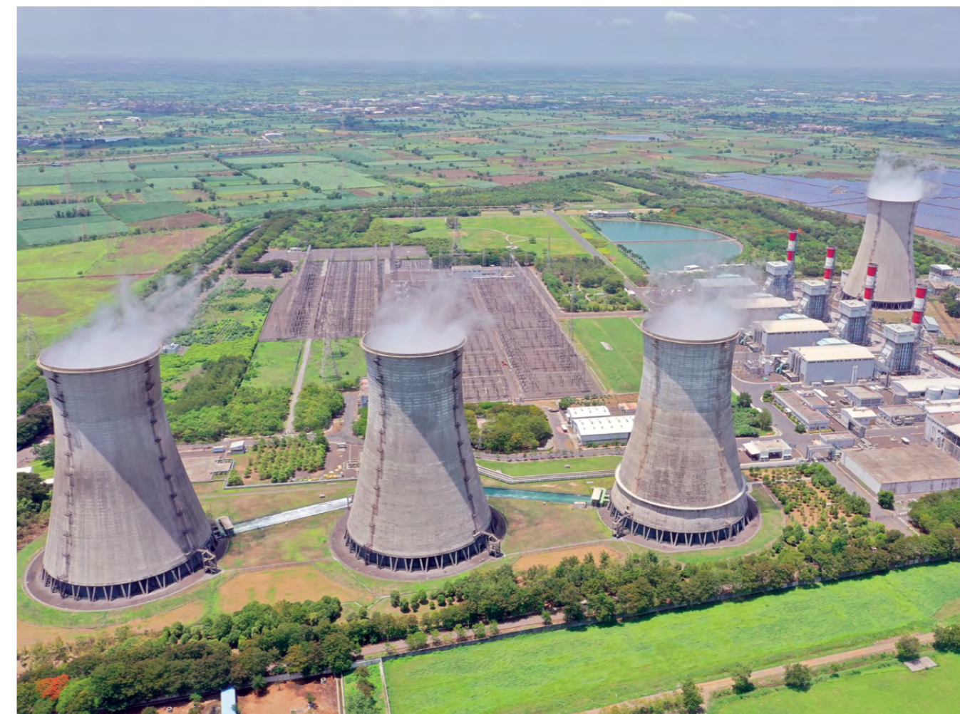
1,147.5 MW SUGEN Plant & 382.5 MW UNOSUGEN Plant at Surat
