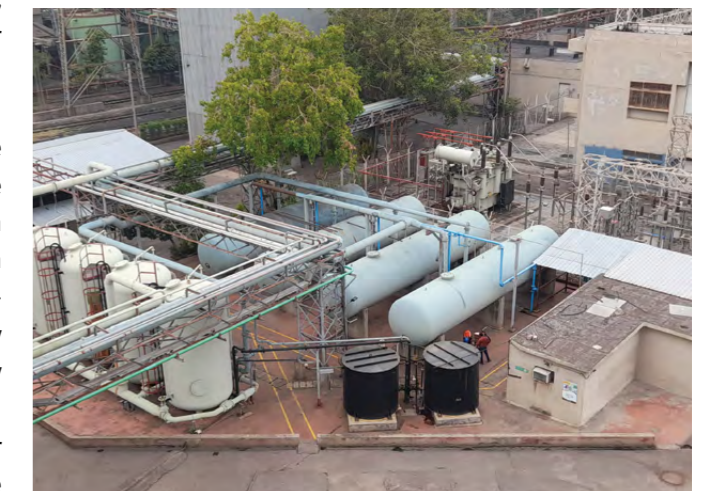
Water treatment plant at AMGEN
