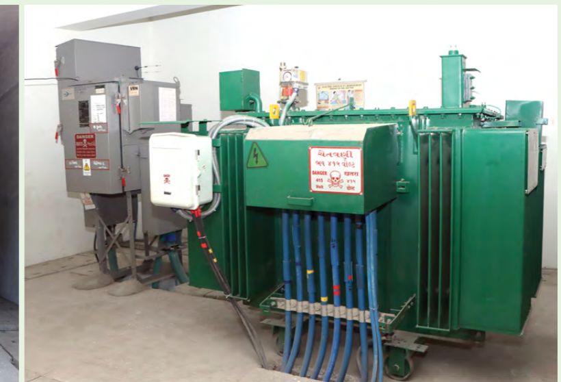
Environment-friendly Hermetically sealed Natural Ester oil filled Distribution Transformer
