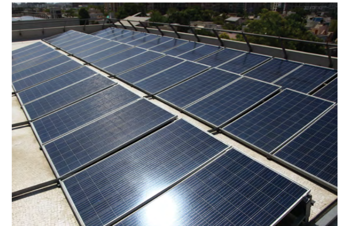
Captive Rooftop Solar System at Corporate
