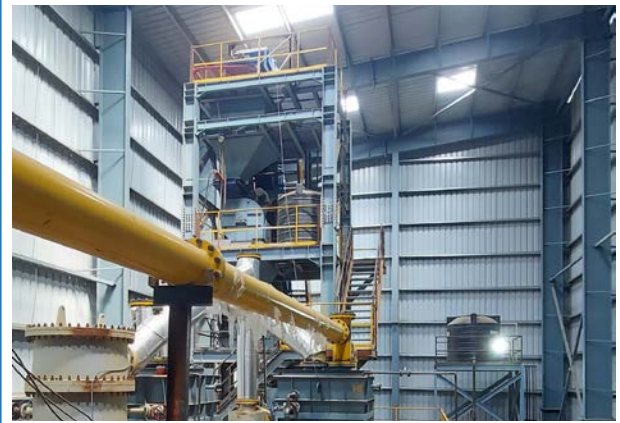
Enhanced Steam Gasification Plant
