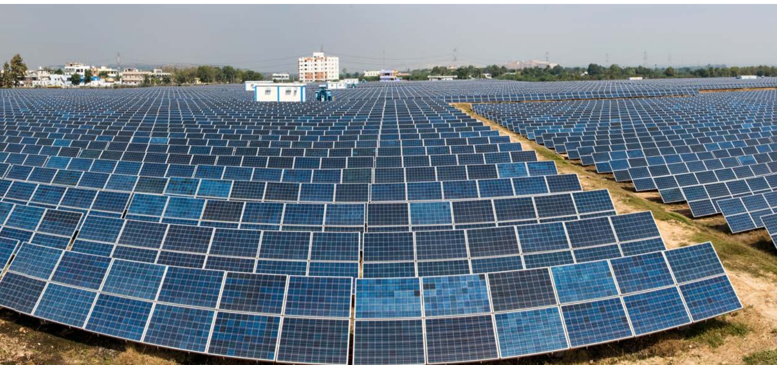
Ramagundam 10 MW Solar PV
