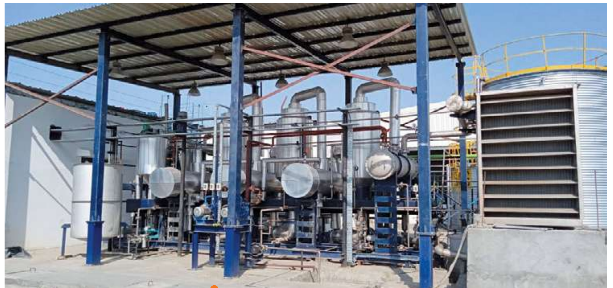
Zero Liquid Discharge (ZLD) Effluent Treatment Plant
