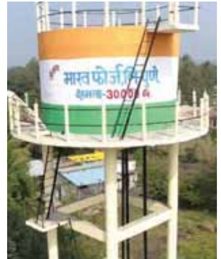
Constructed Drinking Water Tank District: Satara
