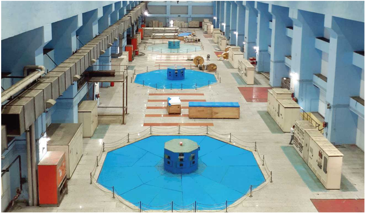
800 MW Parbati-II Project (Himachal Pradesh)- View of Machine Hall
