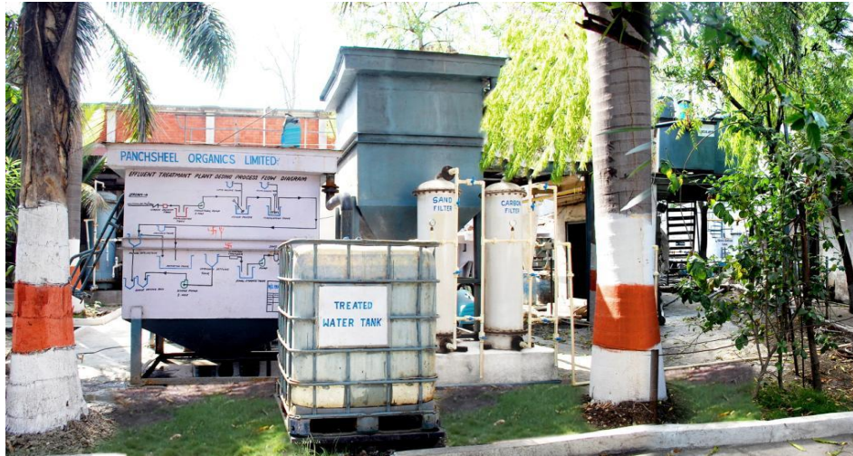
Effluent Treatment Plant
