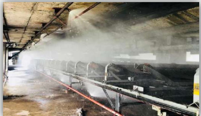
Fig. - Fixed sprinklers along belt conveyor
