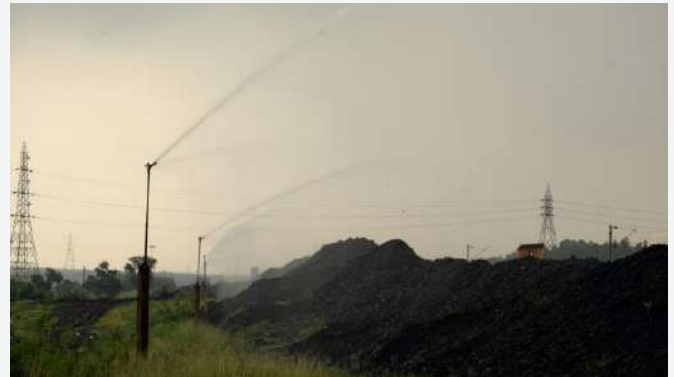
Fig. - Fixed Sprinkler in Belpahad OC, MCL
