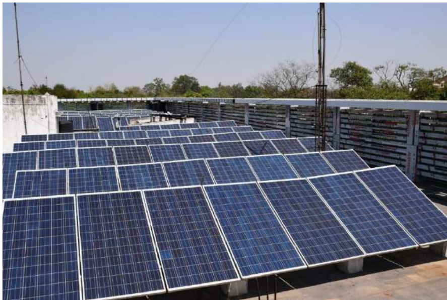
Fig. 70- Roof top Solar plant at CCL
