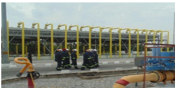
CS - 3 Gas After Cooler
