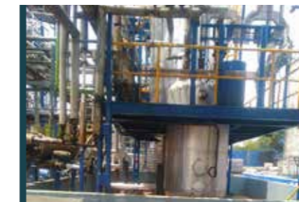
Diketene storage tank with a water curtain for added safety
