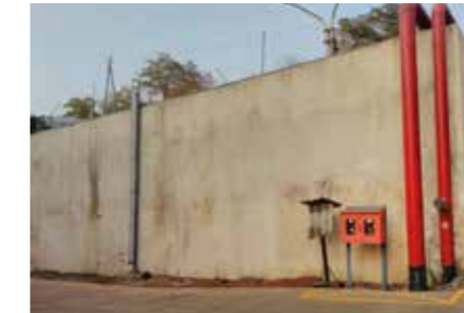
Dedicated water storage tank for fire fighting
