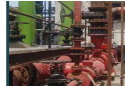
Fire hydrant capacity upgraded with 410 m3 pumping capacity
