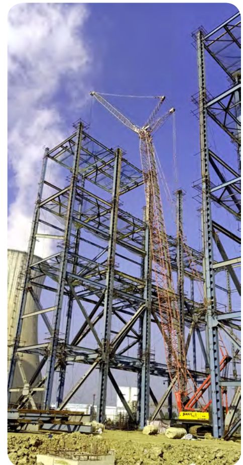
Sany SCC 2500 C (250 MT) crawler crane doing boiler structure erection at BHEL, Rajasthan
