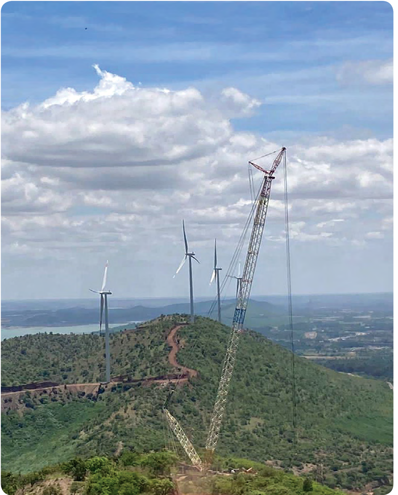
Terex CC2800-1 (600 MT Crane) in windmill configuration handling Nacelle 80 MT at the hub height of 120m Hospete, Karnataka
