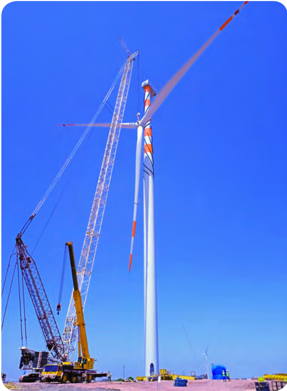
Terex CC2800-1 erecting 2.7 MW Rotor at the hub height of 130M & rotor Dia – 132 `mtrs, turbine model is- 2.7-132 RD in site at Gujarat
