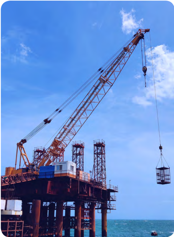
SANY SCC 1500C (150T) main boom 27m placed on jetty for platform erection at Udangudi, Tamil Nadu
