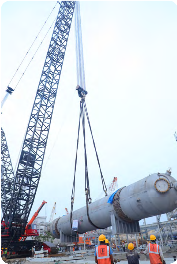
Liebherr LR1800 (1,000 MT Crane) erecting ammonia converter weighing 400 MT during construction of upcoming fertiliser plant in Taloja, Navi Mumbai
