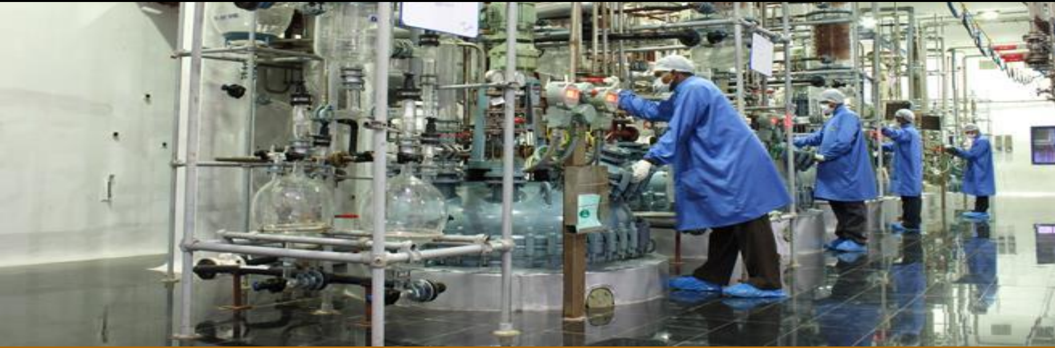
Glass Lined Reactors in Intermediate Area
