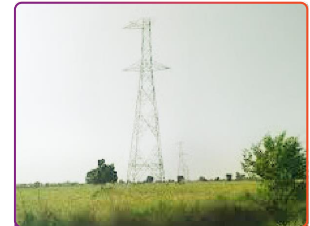
765kV Ghatampur TPS-Agra SC line
