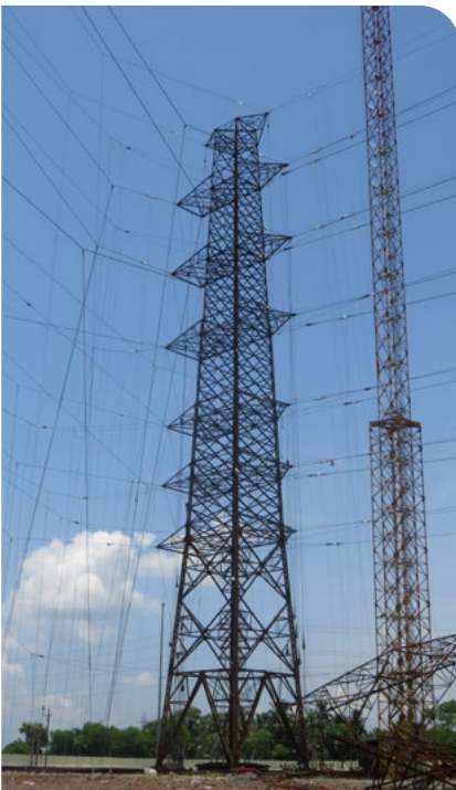
220kV Transmission Tower
