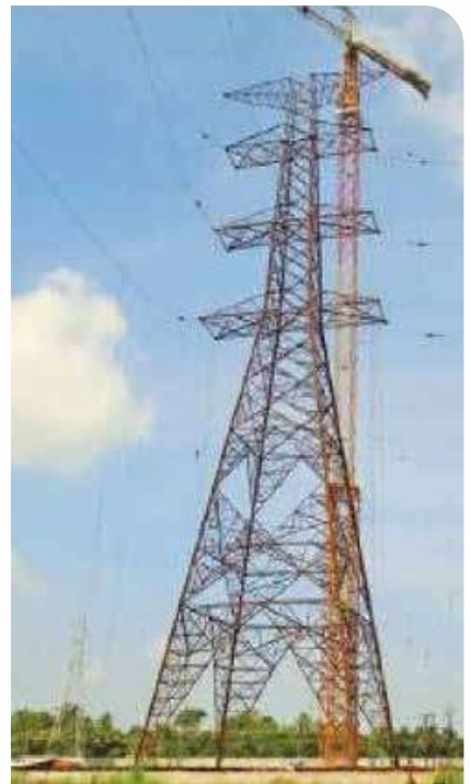
500kV Transmission Tower
