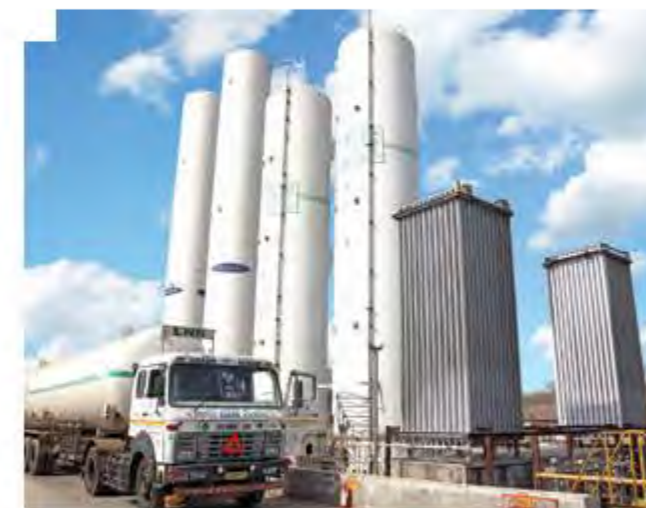
IndianOil, through its Joint Venture Company, IndianOil LNG Pvt. Ltd., has developed a 5-million metric tonnes per annum (MMTPA) capacity Liquefied Natural Gas (LNG) Terminal at Kamarajar Port, Ennore in Tamil Nadu
