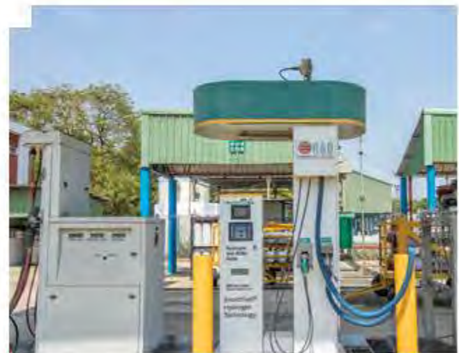
Smart Fuel Hydrogen Technology Station installed at IndianOil R&D Centre at Faridabad, Haryana
