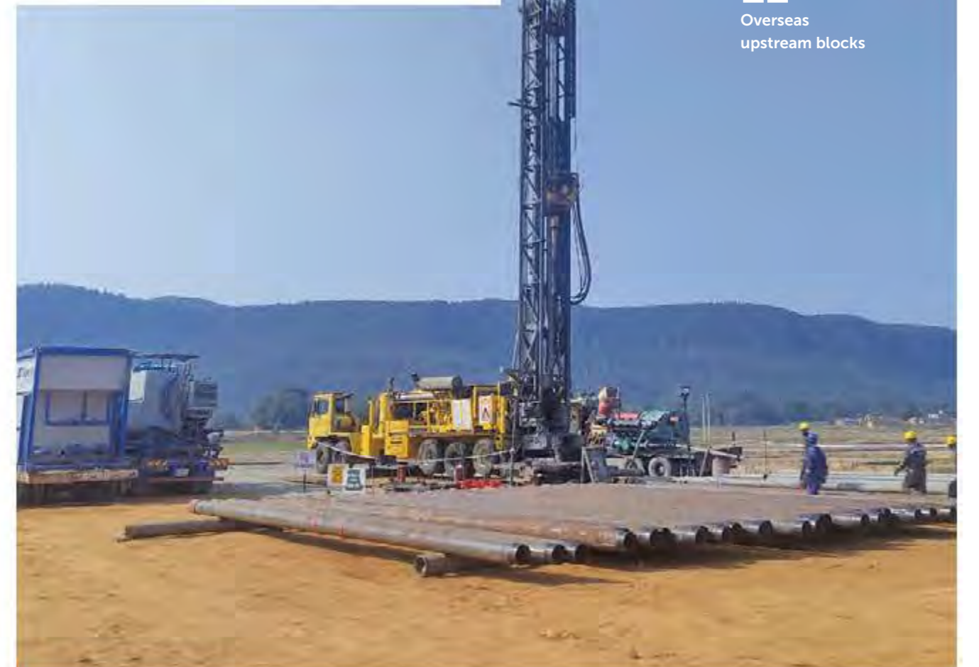
Ongoing operations at well no. BR-51 in the Coal Bed Methane (CBM) Block, Jharkhand
