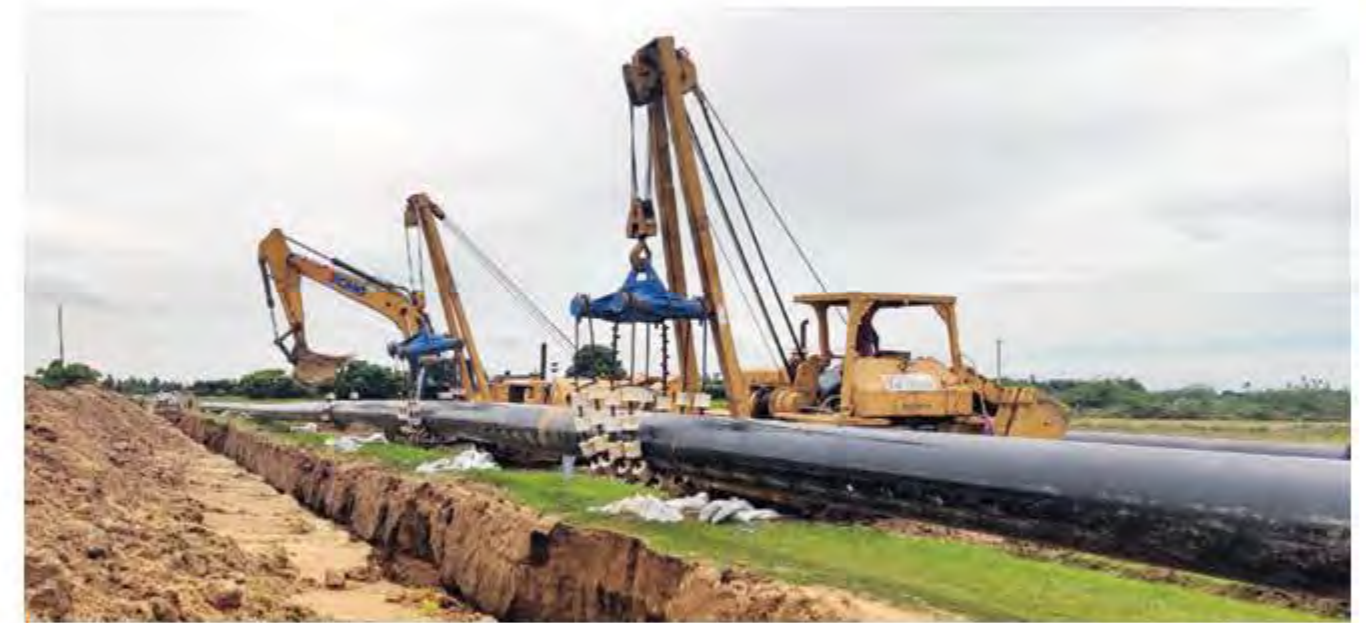
IndianOil's Pipeline infrastructure has expanded with the completion of the 1200 Km-long Paradip-Hyderabad product Pipeline
