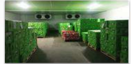
Cold Storage unit (Sangola)
