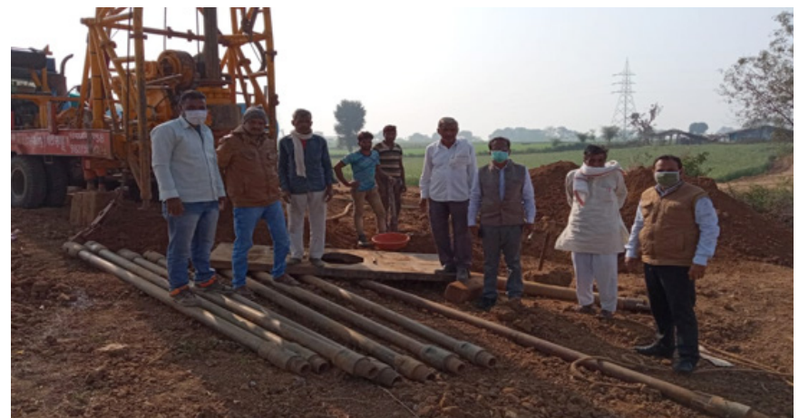
Borewell & Hand pump at a neighboring village in Budhni, Madhya Pradesh
